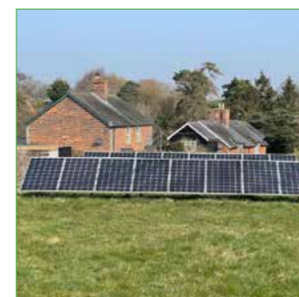
Small domestic ground-mounted array of photovoltaic panels on Bury Road
